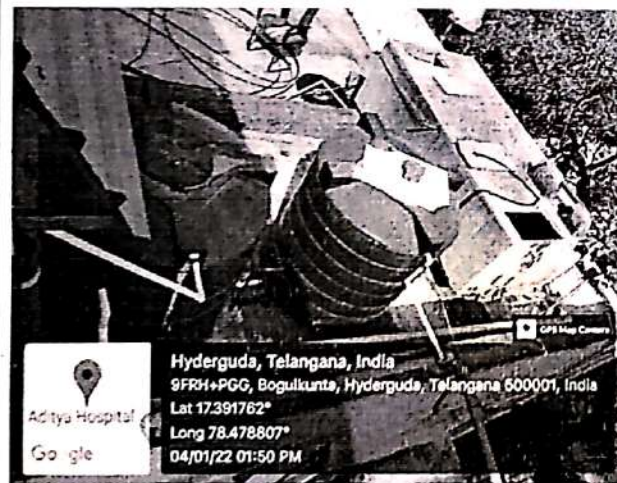
Over Head tank at B Block
