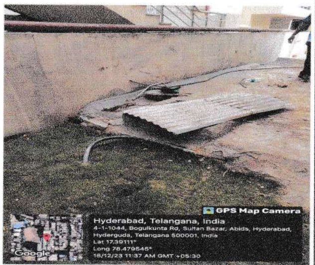
Waste water collection Pit , used for plants
