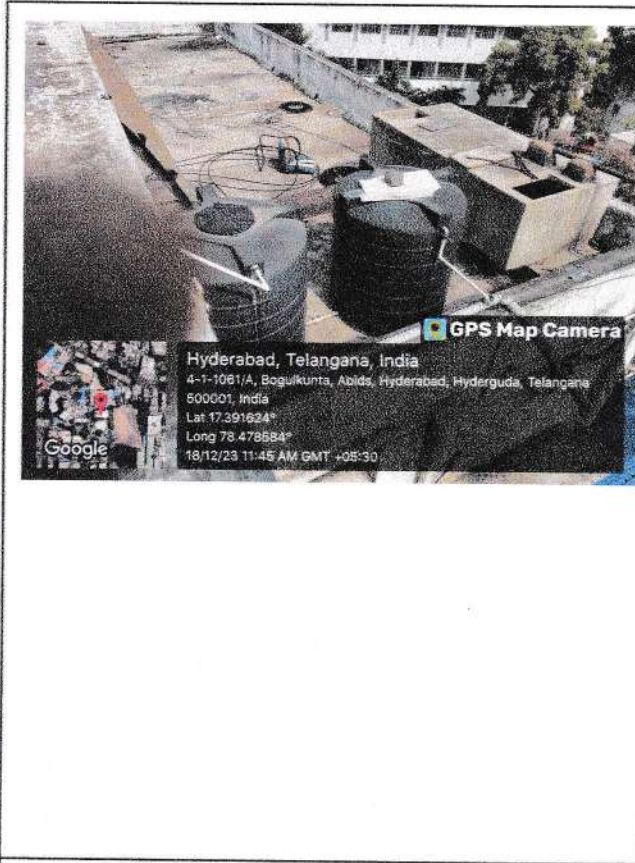
Overhead tank with Distribution of Water
