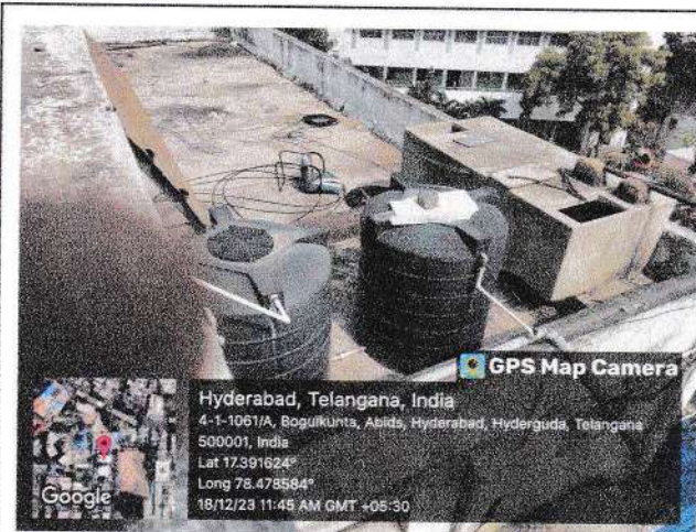
Over Head tank at B Block
