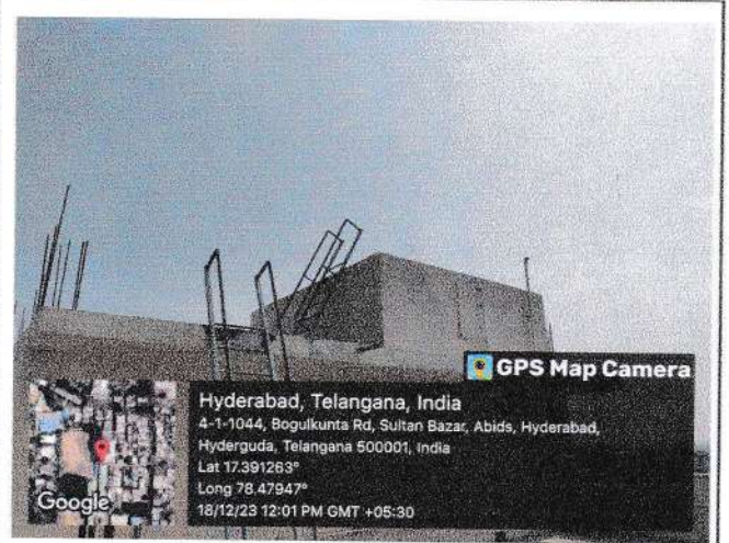
Storage Tank for Drinking water at E Block
