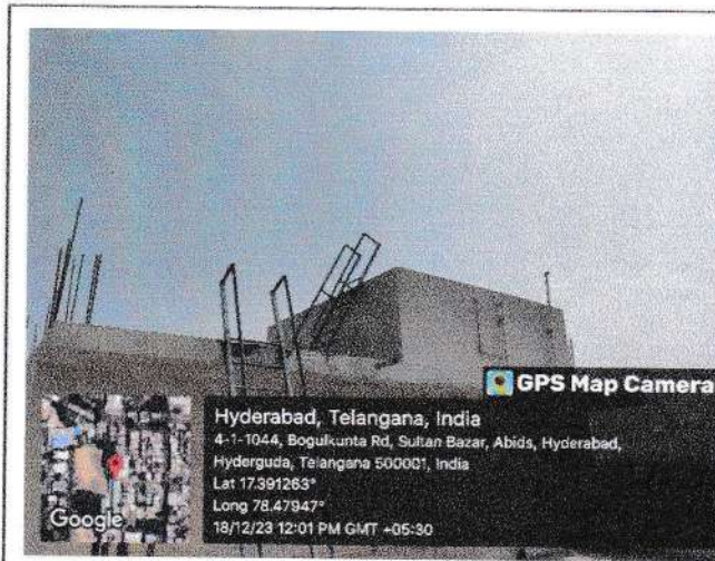
Over Head tank at E Block
