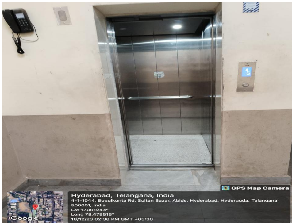
Lift in 'E' block
