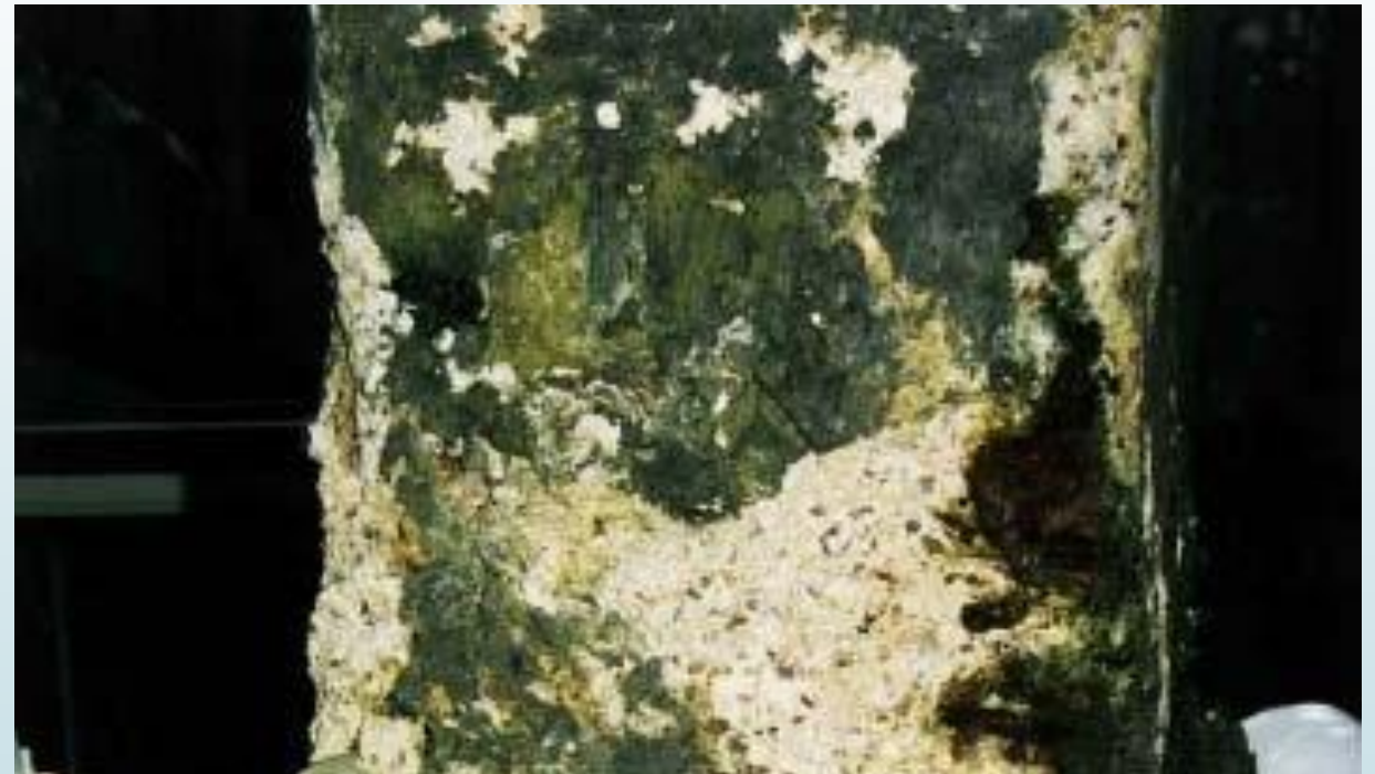
Fig. 37. Deterioration due to chemical action - Sulphate Attack
