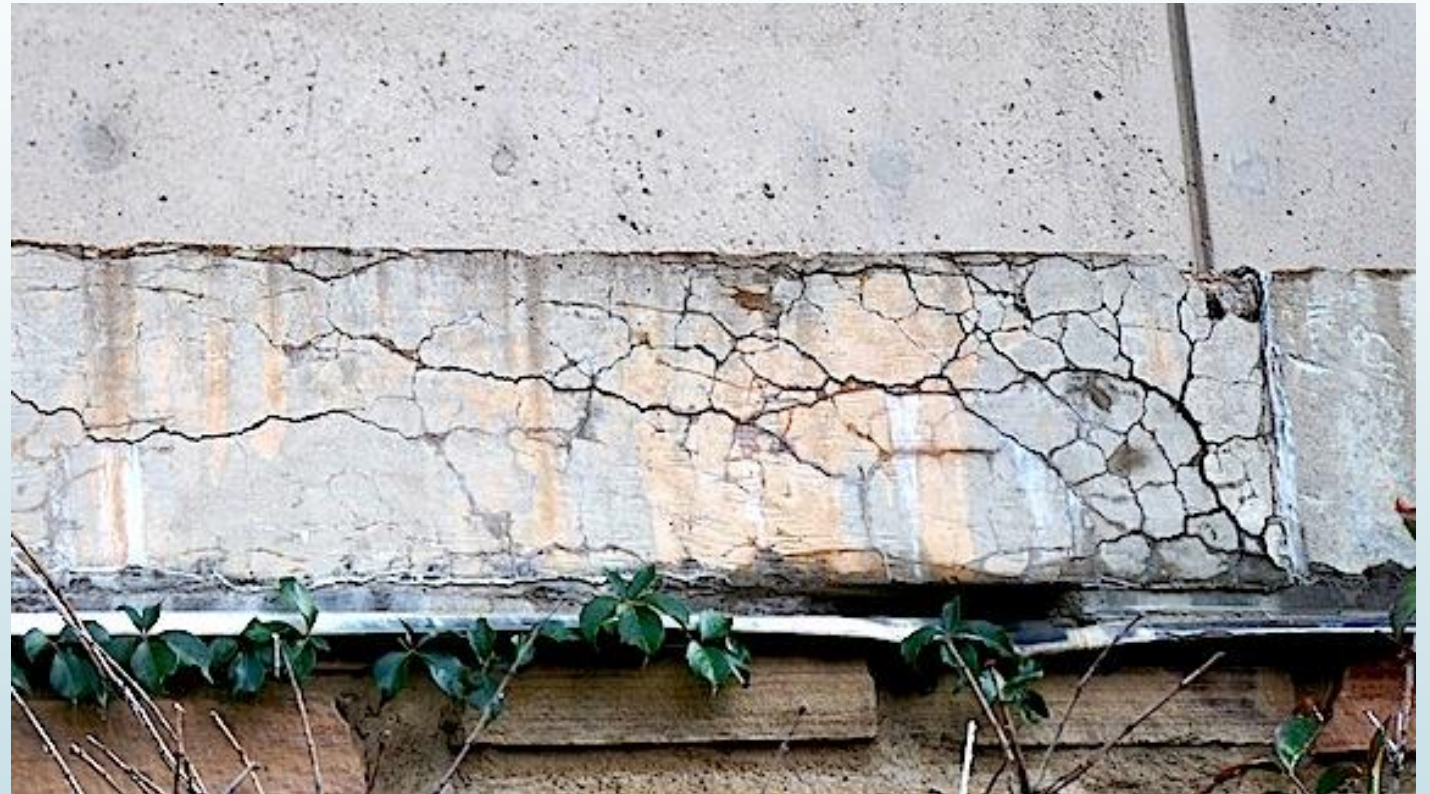
Fig. 34. Cracks Pattern due to chemical action – Possibly Alkali Aggregate Reaction (AAR)
