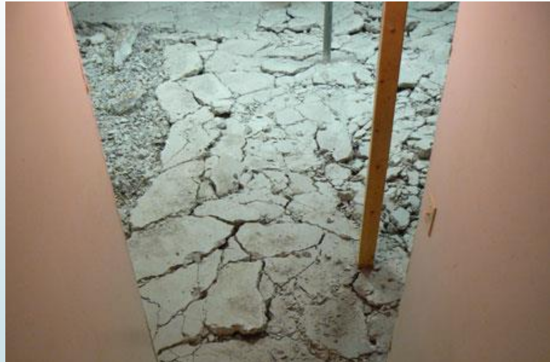
Fig. 36. Cracks Pattern due to chemical action – Sulphate Attack
