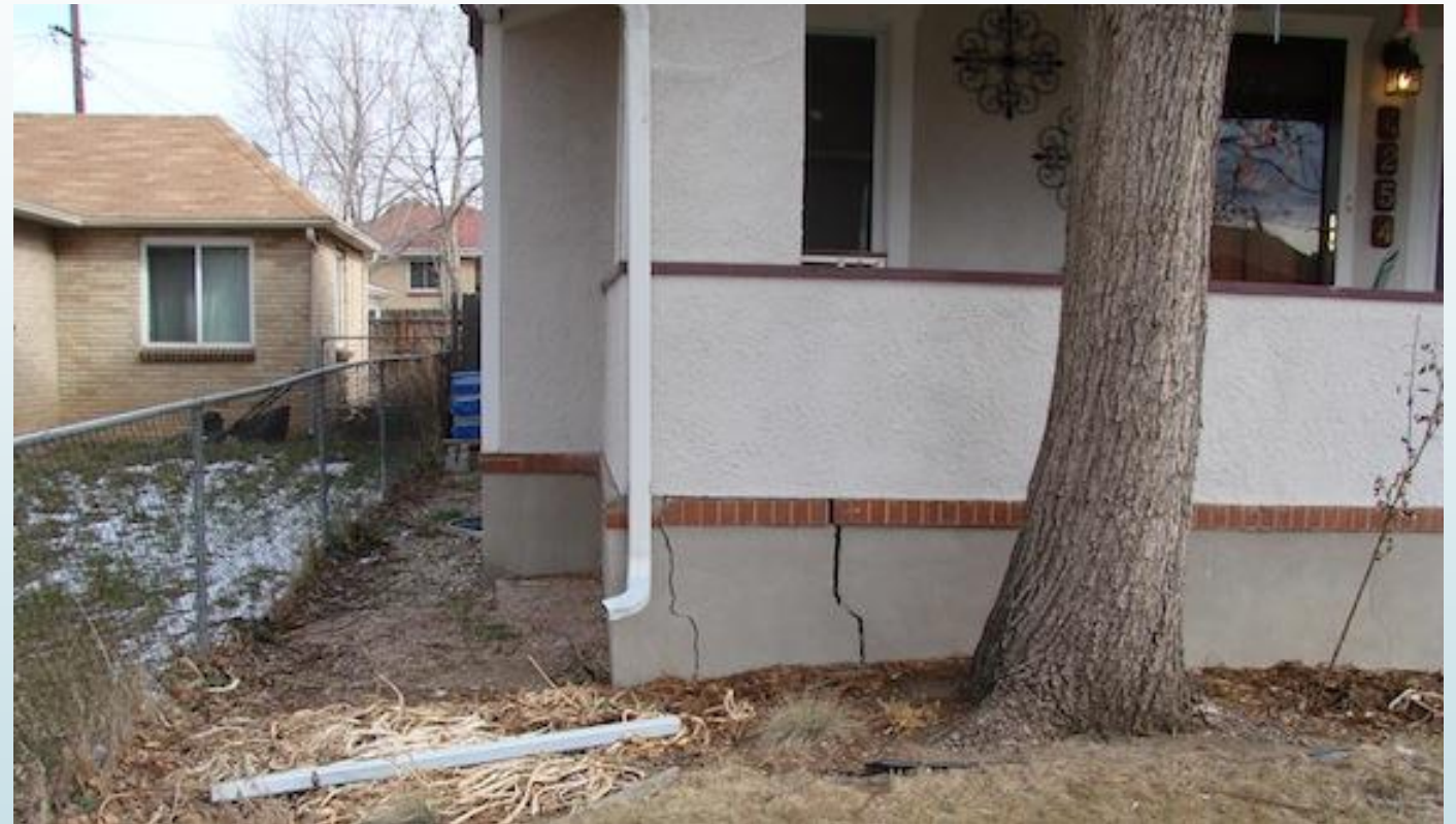
Fig. 33. Masonry cracks due to Differential Settlement
