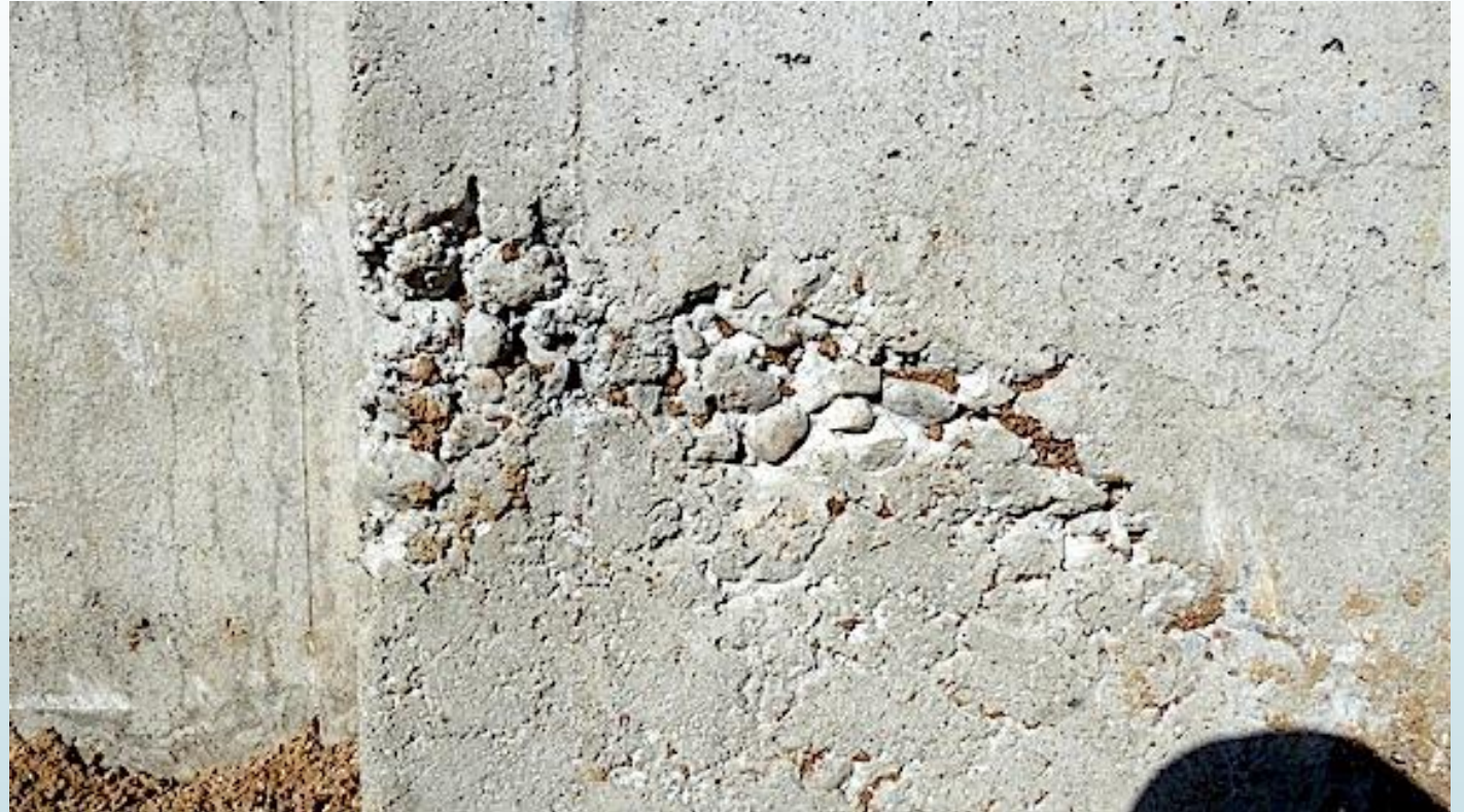
Fig. 23. Honey-combing due to improper consolidation
