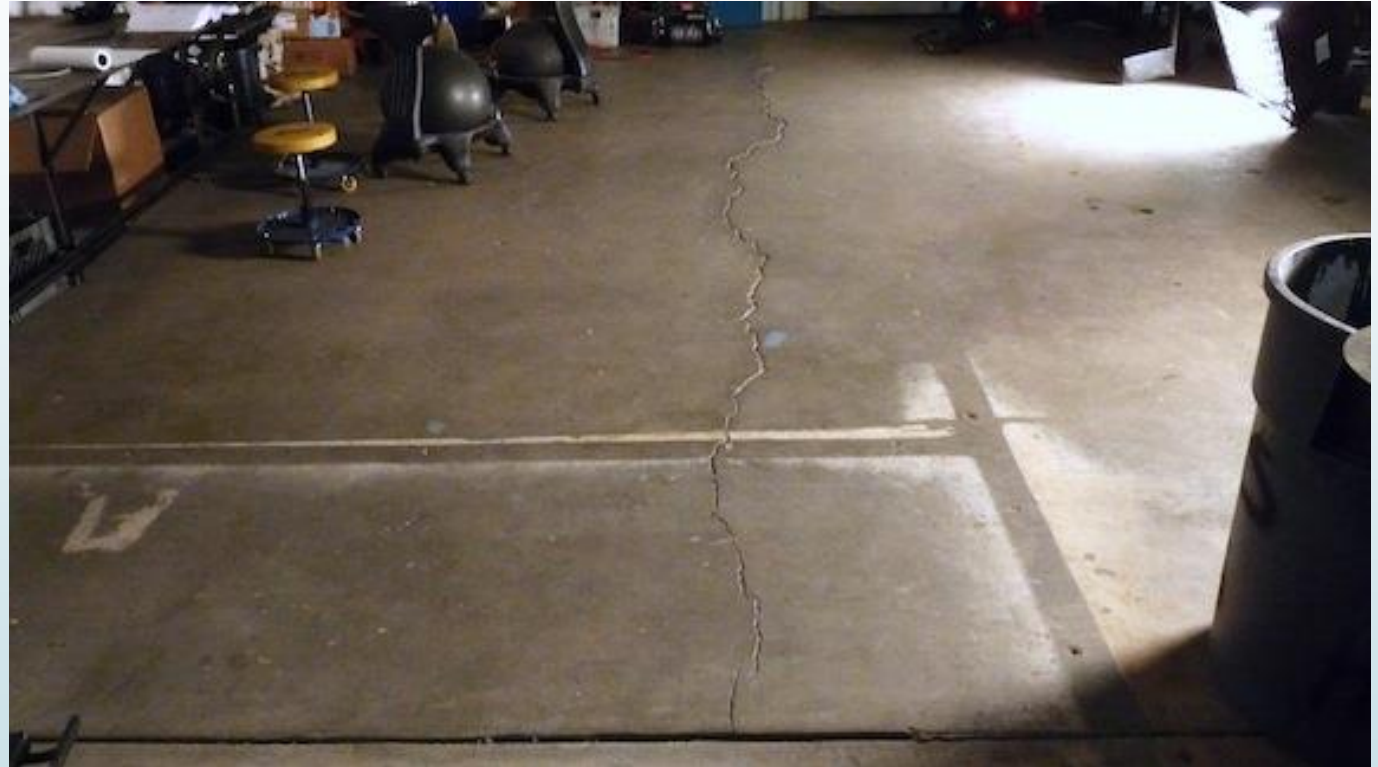
Fig. 26. Drying Shrinkage Cracks
