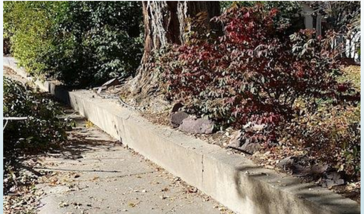
Fig. 31. Creep with cracks
