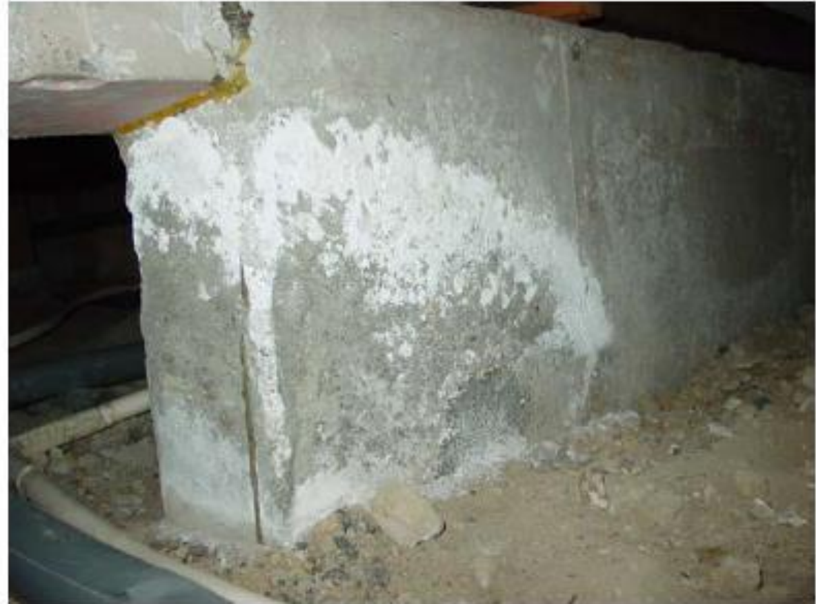
Fig. 35. Damage Pattern due to chemical action - Sulphate Attack
