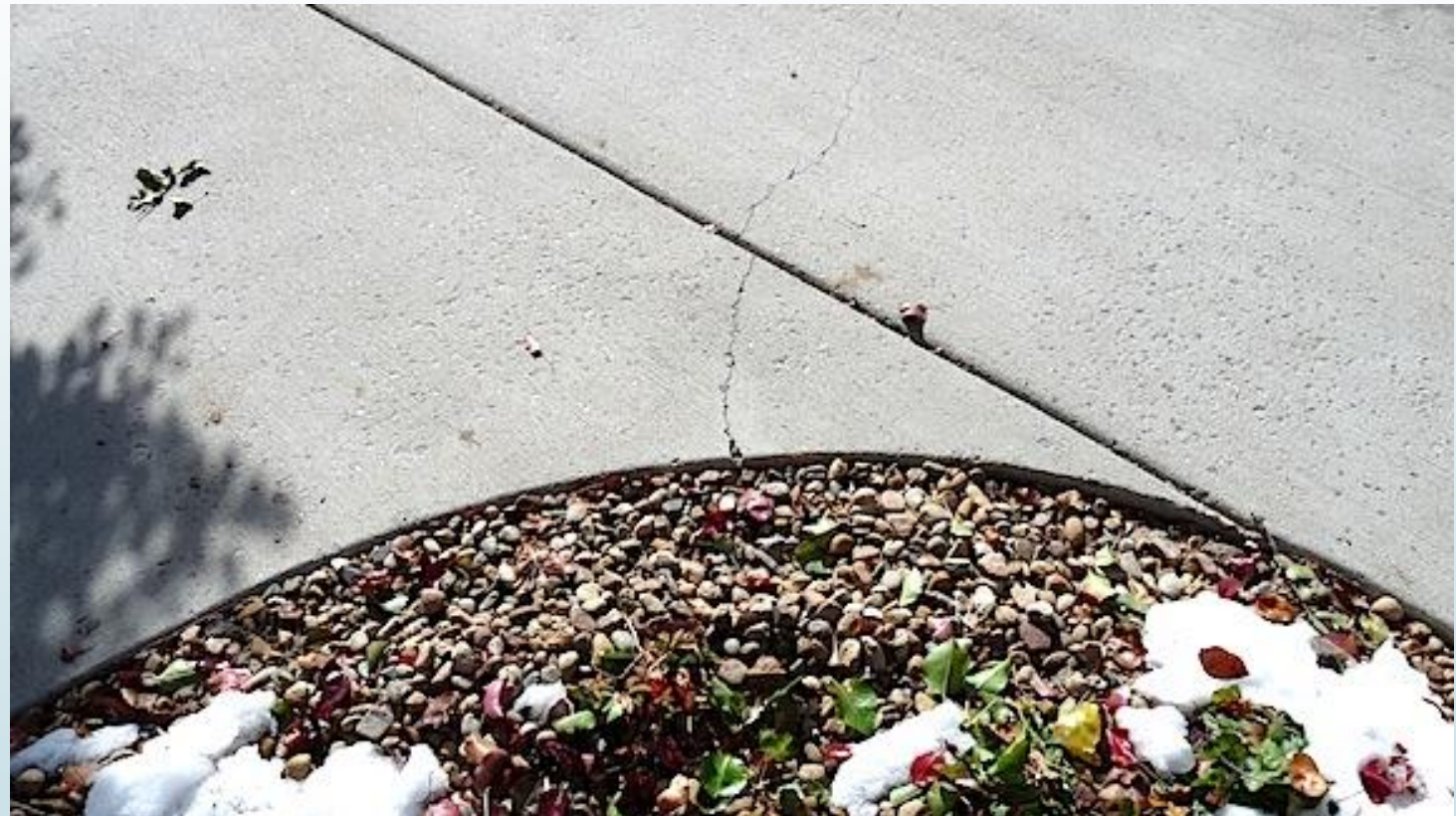
Fig. 30. Re-entrant corner cracks
