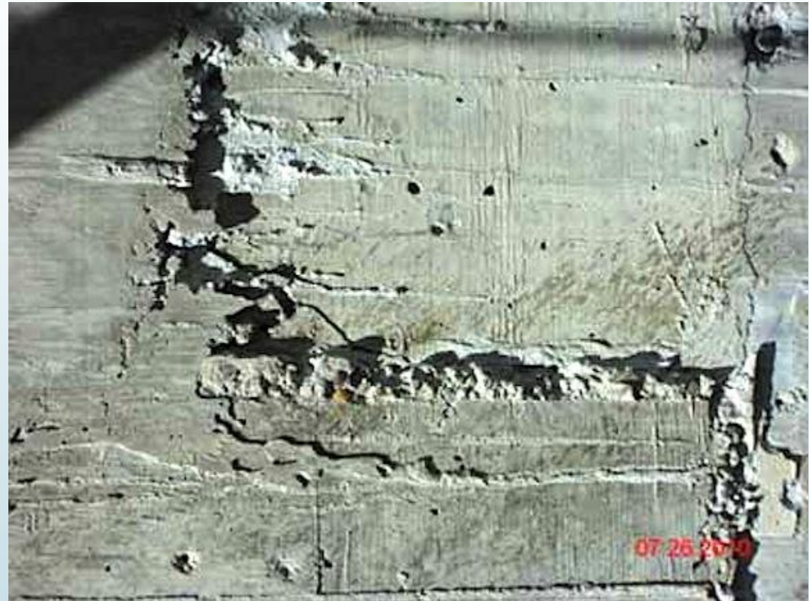
Fig. 22. Cold Joint in Concrete
