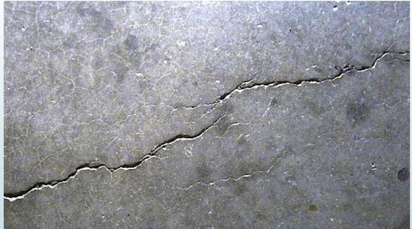
Fig. 27. Drying Shrinkage Cracks (Discontinuous)
