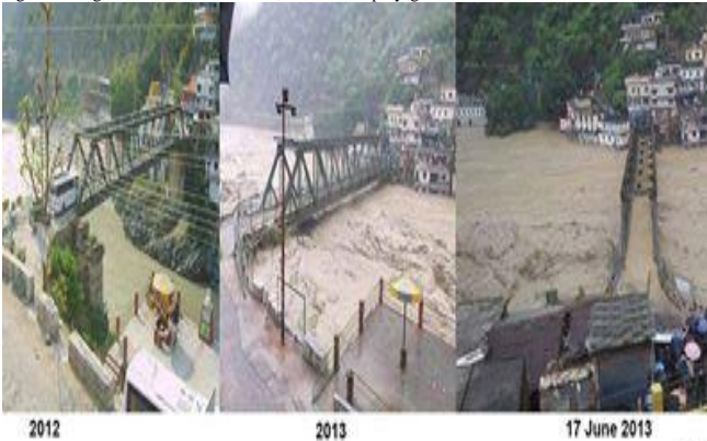
Fig. 8–Damaged Bridge in Uttarkashi Town in June 2013
